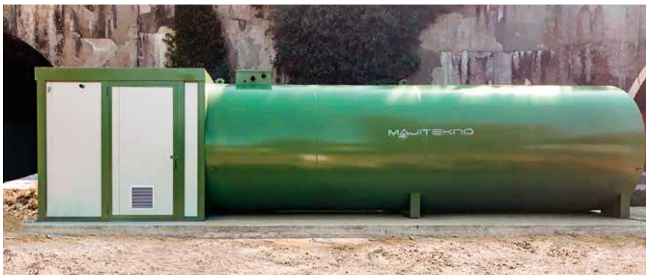
MF CO-TBI special - Motorway tunnel - Florence
