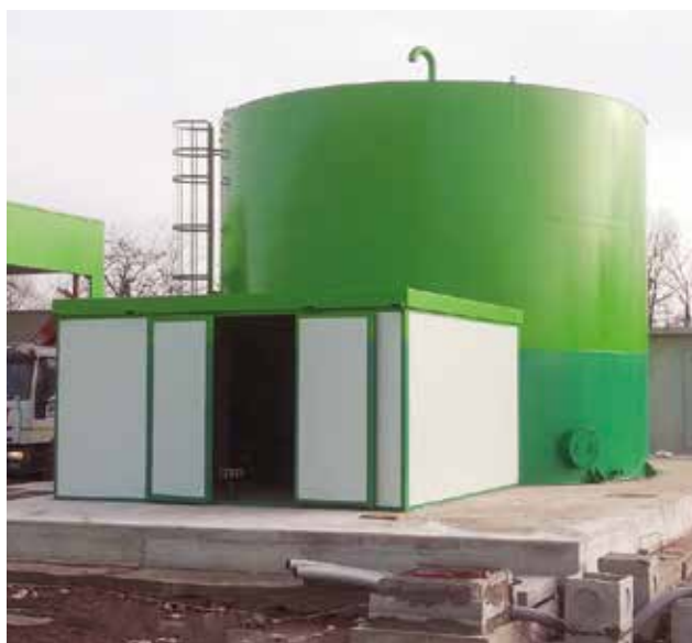
MF CO-TW 250 m³ + TBOX - Plastic recycling plant - Biella
