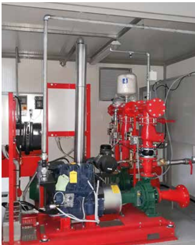
Fire pump room interior
