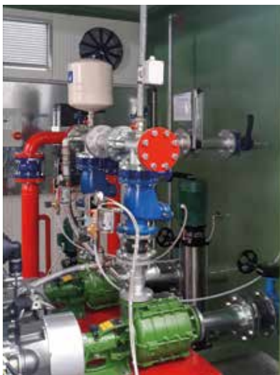
MF CO-TBI - Motorway tunnel system - Florence
