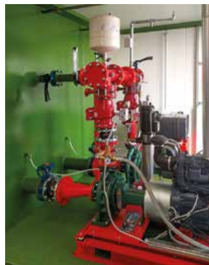
MF CO-TBI - Biogas plant - Brescia
