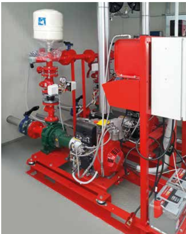
Fire pump room interior
