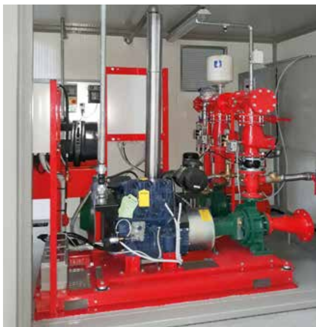
Fire pump room interior
