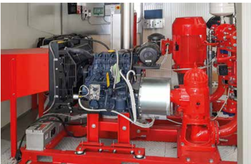
Fire pump room interior
