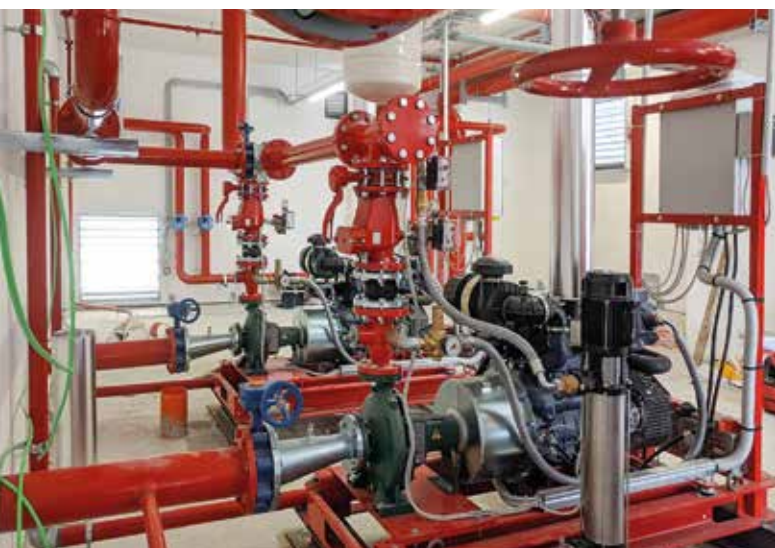
MF CO-TW 1800 m³ + TBOX - Logistics centre - Novara
