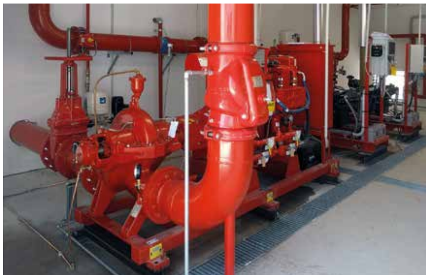
MF CO-TW 1800 m³ + TBOX - Logistics centre - Novara
