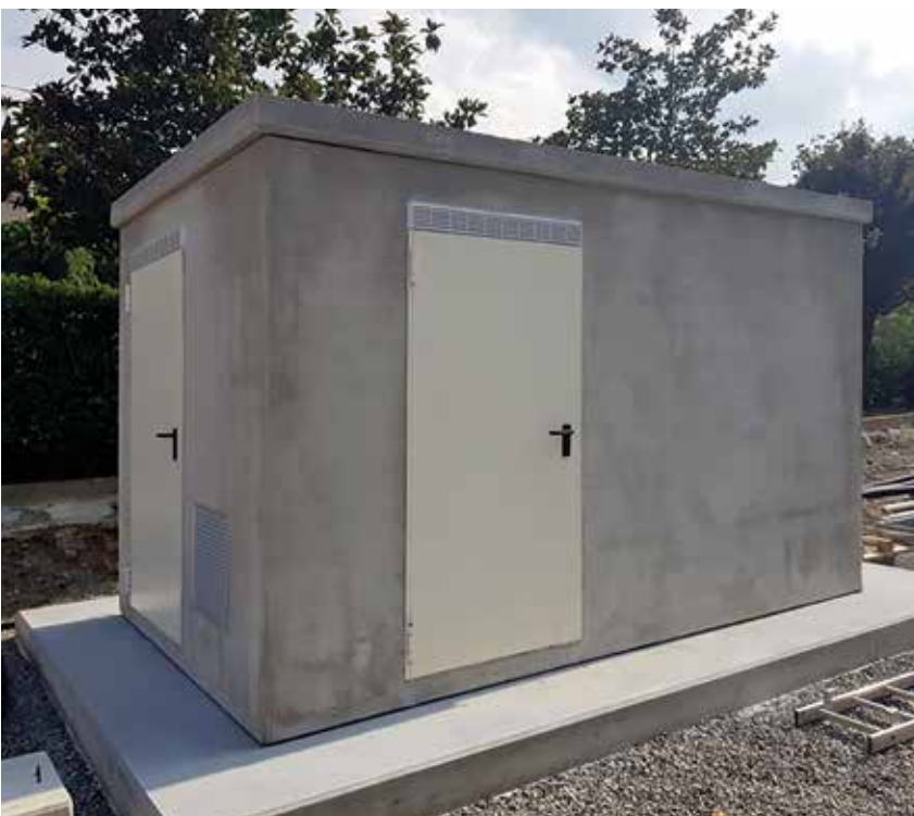
External technical fire pump room in reinforced concrete
