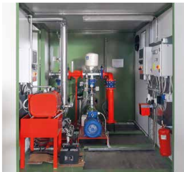
MF CO-TBI special - Motorway tunnel - Florence
