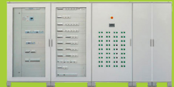
Power Center Panel
